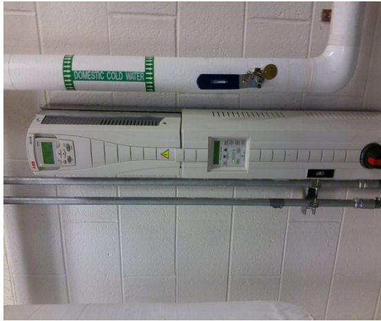
New controller for variable speed pump GOB
