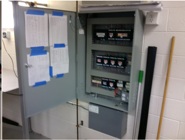
Local control center GOB heat and ventilation
